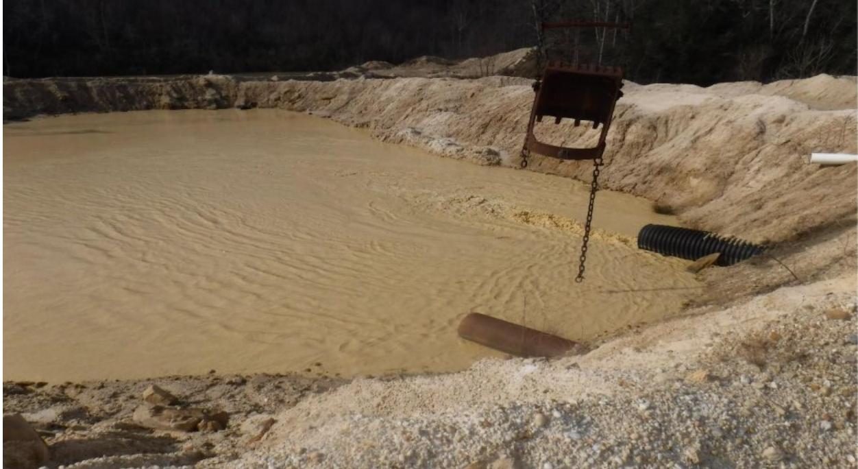
Photo 9 – Process wastewater treatment cell 2 inlet pipe.
