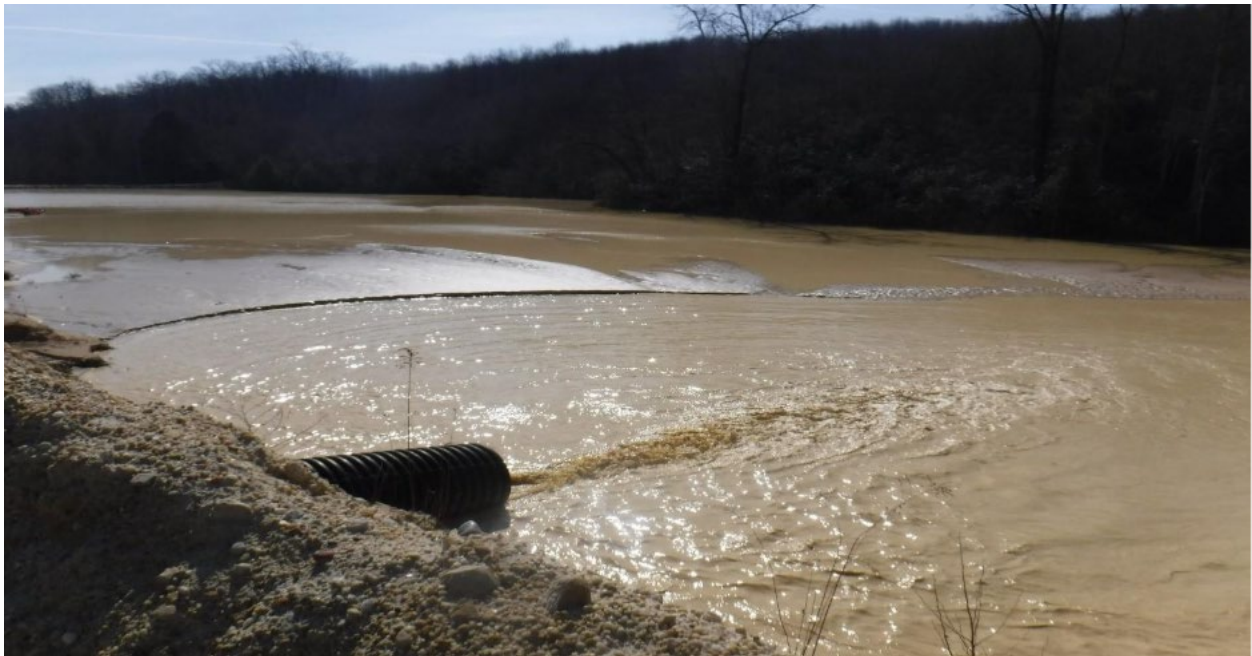
Photo 10 – Outlet of process wastewater cell 2 discharging into upper pond.
