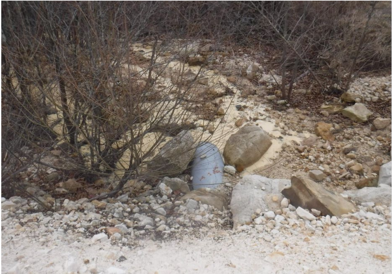
Photo 14 - NPDES Permit outfall 01J00062003.
