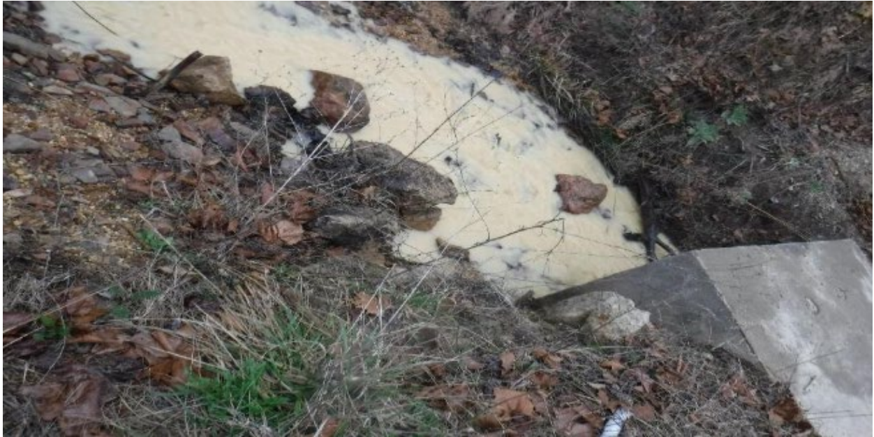
Photo 1 - Process wastewater discharged from Ohio Sands LLC entering road culvert to Jackson Lake.
