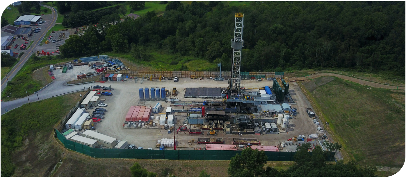
Fracking infrastructure in Wayne, Ohio. Photo by Ted Auch, FracTracker Alliance.
